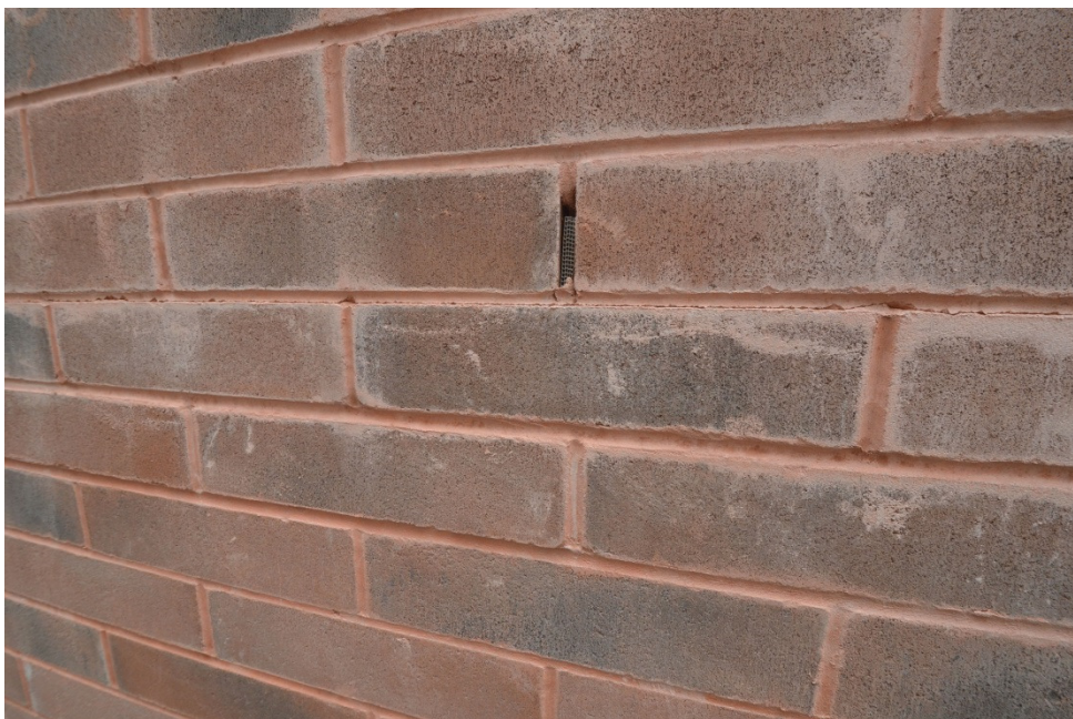
This mortar was tooled too early. Mortar smears and gaps at the bond line can occur.
