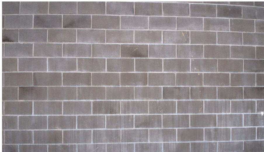
This wall was over 100 degrees when the detergent was applied- flash set
